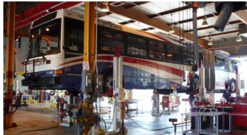
43,000 lb bus, 6 mobile lifts, 16,000 lb capacity each lift
